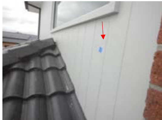
Rear garage- Saw blade mark
