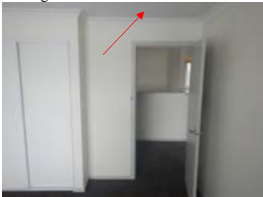
Ceilings out of level
