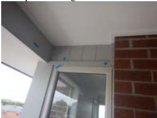
Nail holes to cladding not filled with a paint filler prior to paint
