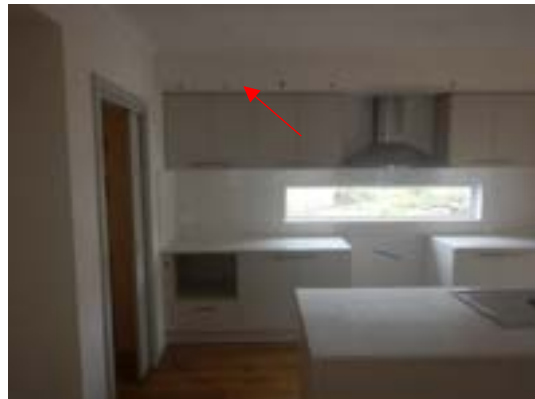
Bulkhead out of level
