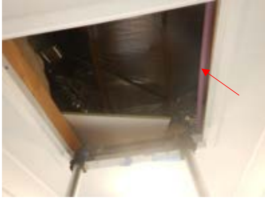
Water pipe interfering with manhole lid
