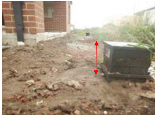
Pit to be adjusted to landscaping height, currently non-functioning
