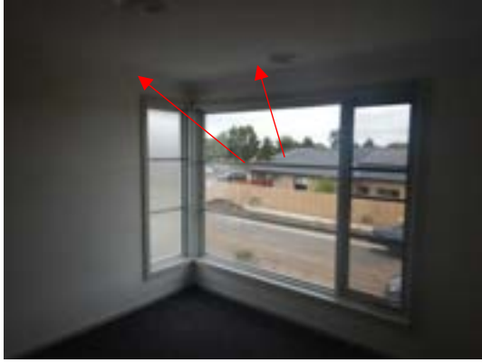
Ceilings out of level
