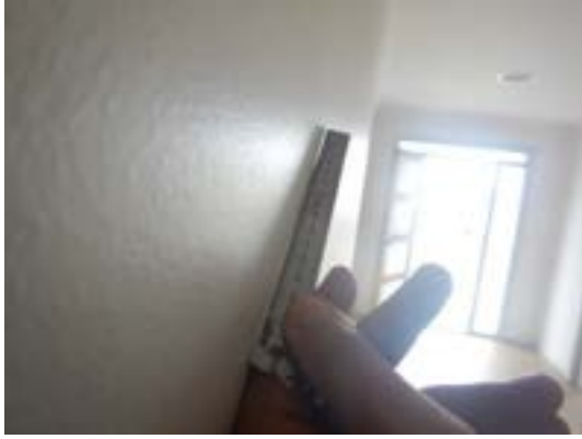
Bulge in plaster.
