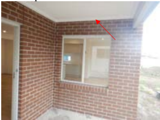
Ceiling out of level
