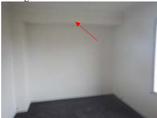
Guest-Bulkhead out of level
