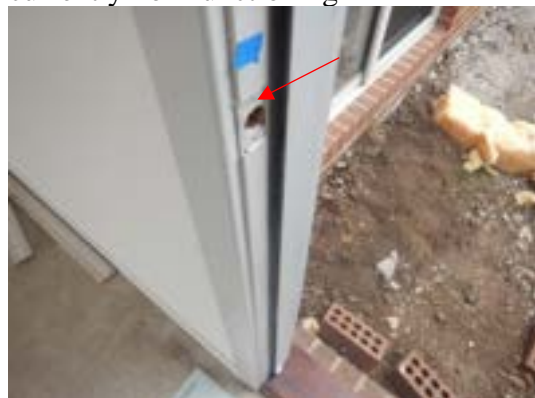
Missing striker plates
