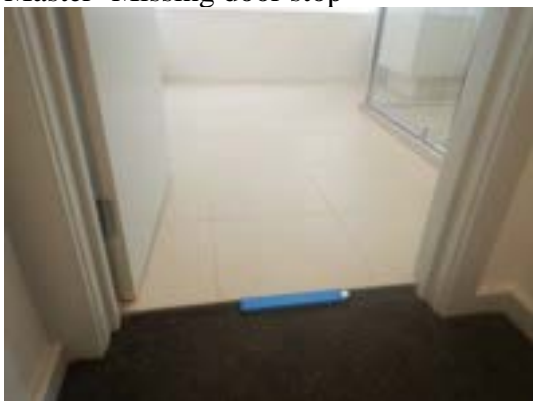
Transition strip required due to step between tiles and carpet
