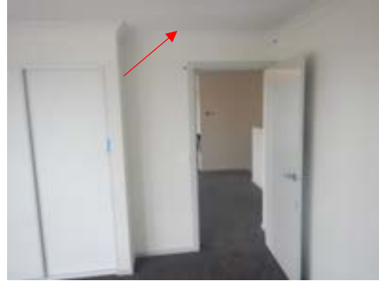
Ceilings out of level
