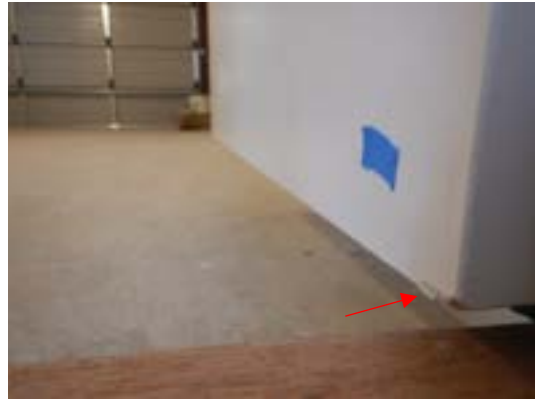
Lack of sanding to doors, rough door edges throughout
