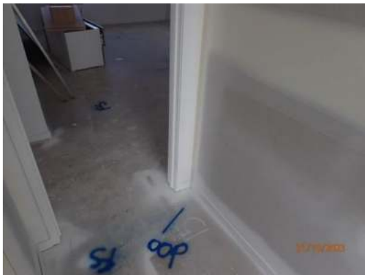
Bed 2 – out of plumb
