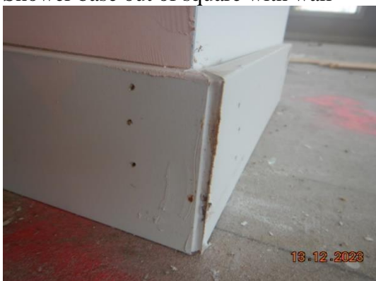
Poor fixing finishes throughout
