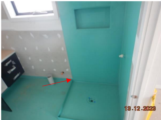
Shower base out of square with wall
