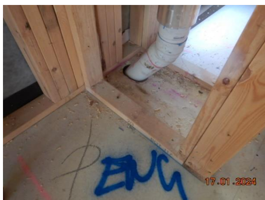
Slab appear to have been altered to riser
