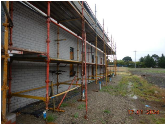
Unable to inspect external due to scaffolding. To be checked at next stage.
