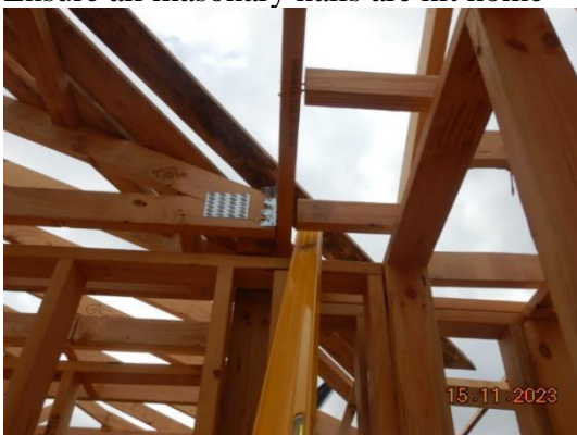
Valley boards throughout have not been securely fixed to trusses
