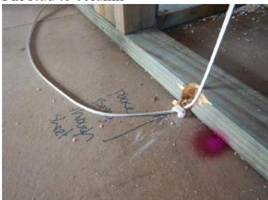
Wire protruding wall
