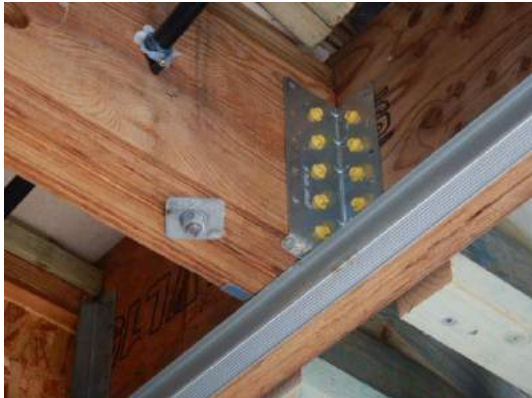
Missing screws to Split hanger
