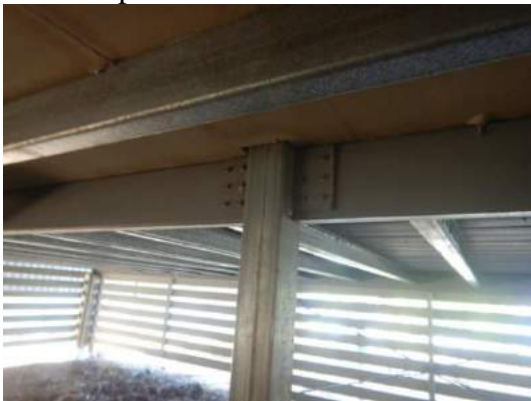
Beam to post missing tech screws
