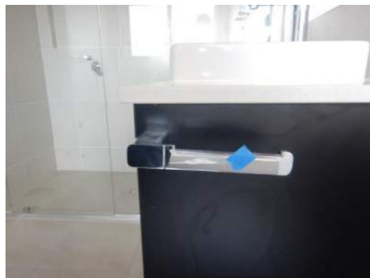
Loose Toilet Roll holder
