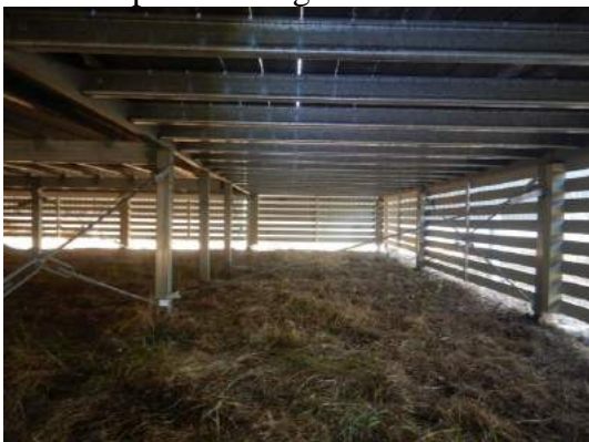
Appears missing Brace section
