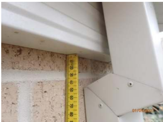
Fascia out of level & alignment with bed joint
