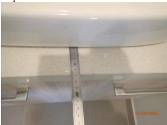
Caulking incomplete through
