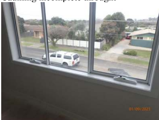
Master – service window cannot open
