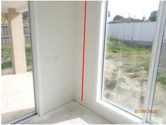
Out of plumb
